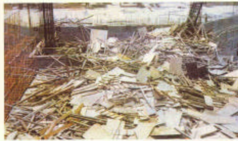
Storm damage to the formwork of a shed and a storage shed that had almost been completed.
